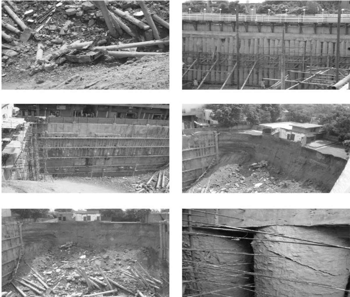
Fig.1(a). Design failure sites.
